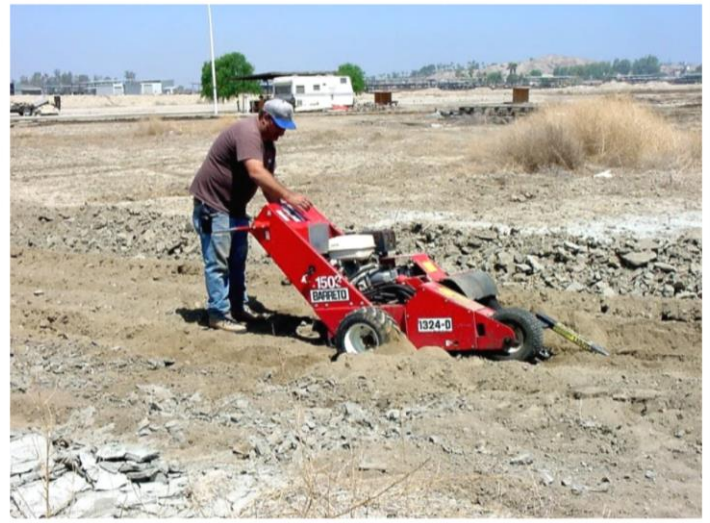
Dave Hollingworth operating a Ditch Witch, digging a trench for running electric and water lines to the relocated runway in June 2002.
