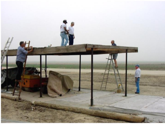
Members putting up a Pit Shade Structure at the relocated Runway in May 2002.
