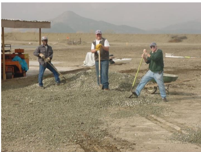
Roy Truitt, Jeff Vanderpol, and Mel Santmyers spreading gravel in the parking area of the relocated runway on February 14, 2003.
